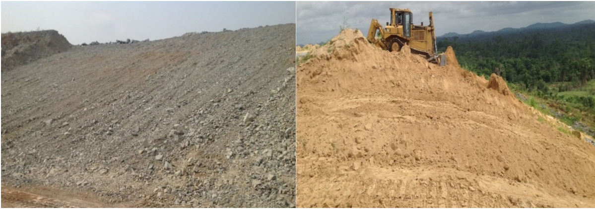
Figure 2: The graded waste-rock dump (left); replacement of the STS on the graded rocks (right).
