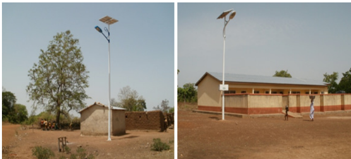
Figure 9: Solar street lighting systems (SSLs) installed at Kataah community center and clinic in the Wa East district.
