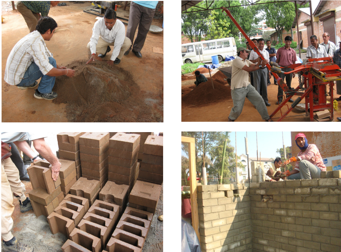
Figure 4. CSEB production: Mixing of soil, compression in the Auram3000 machine, laying for curing and laying the blocks in the wall
